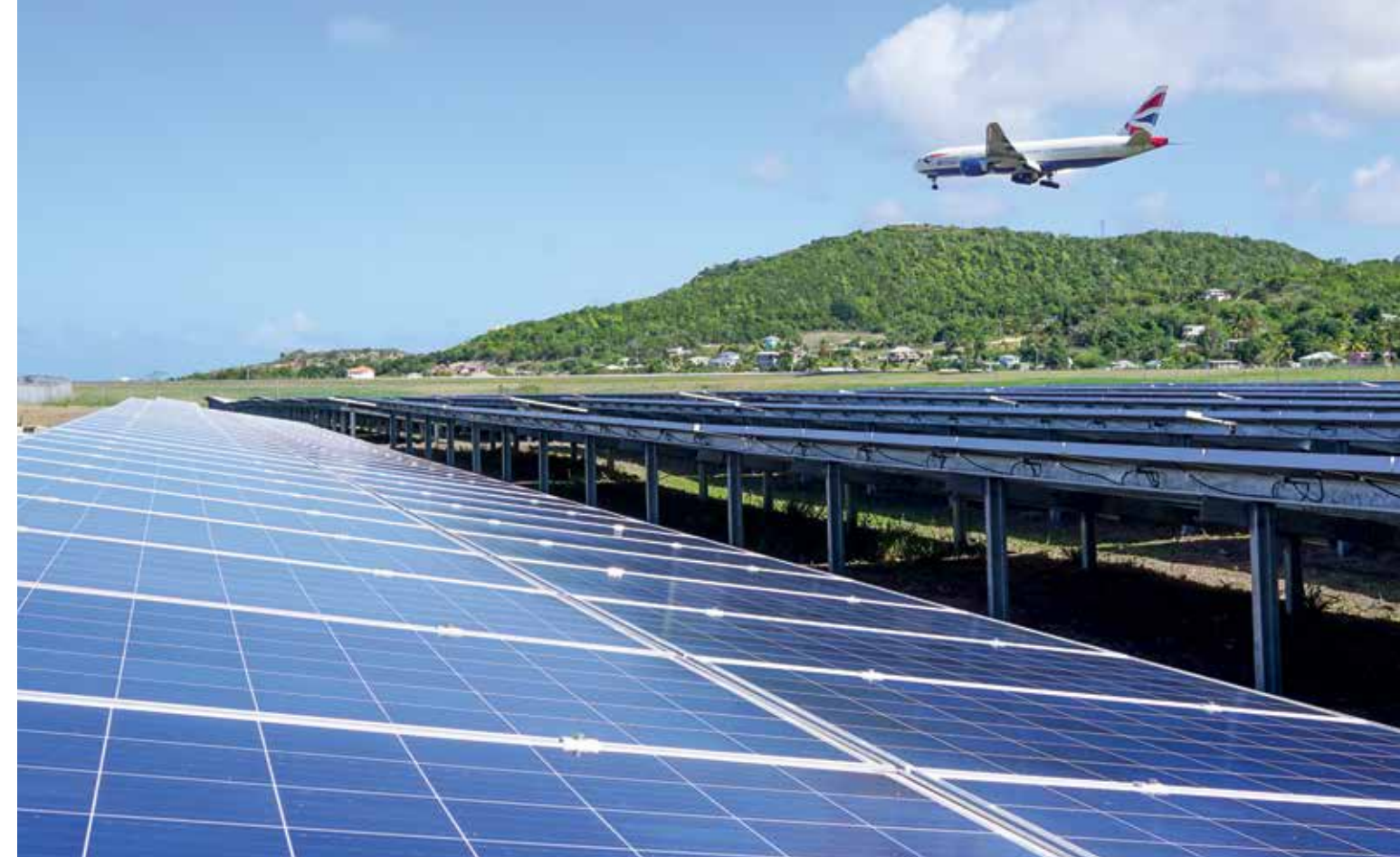
Solar panels in Antigua and Barbuda. Source: Found on Meeco.net by The Meeco Group
